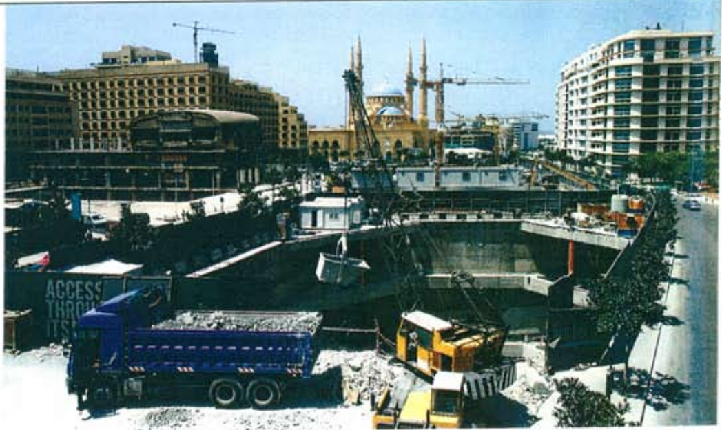
Labourers work at a construction site of Solidere, in downtown Beirut. REUTERS/Sharif Kam
